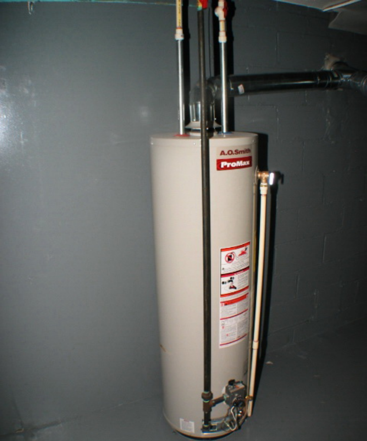
11058 Lakepointe After: Hot water
