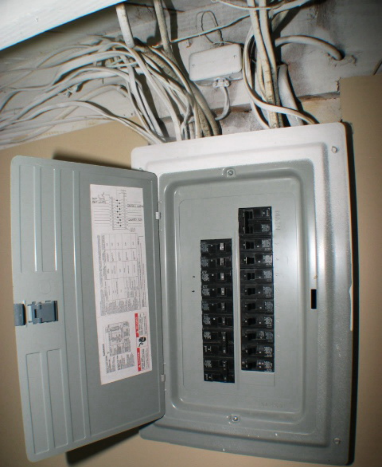
11058 Lakepointe After: Electrical
