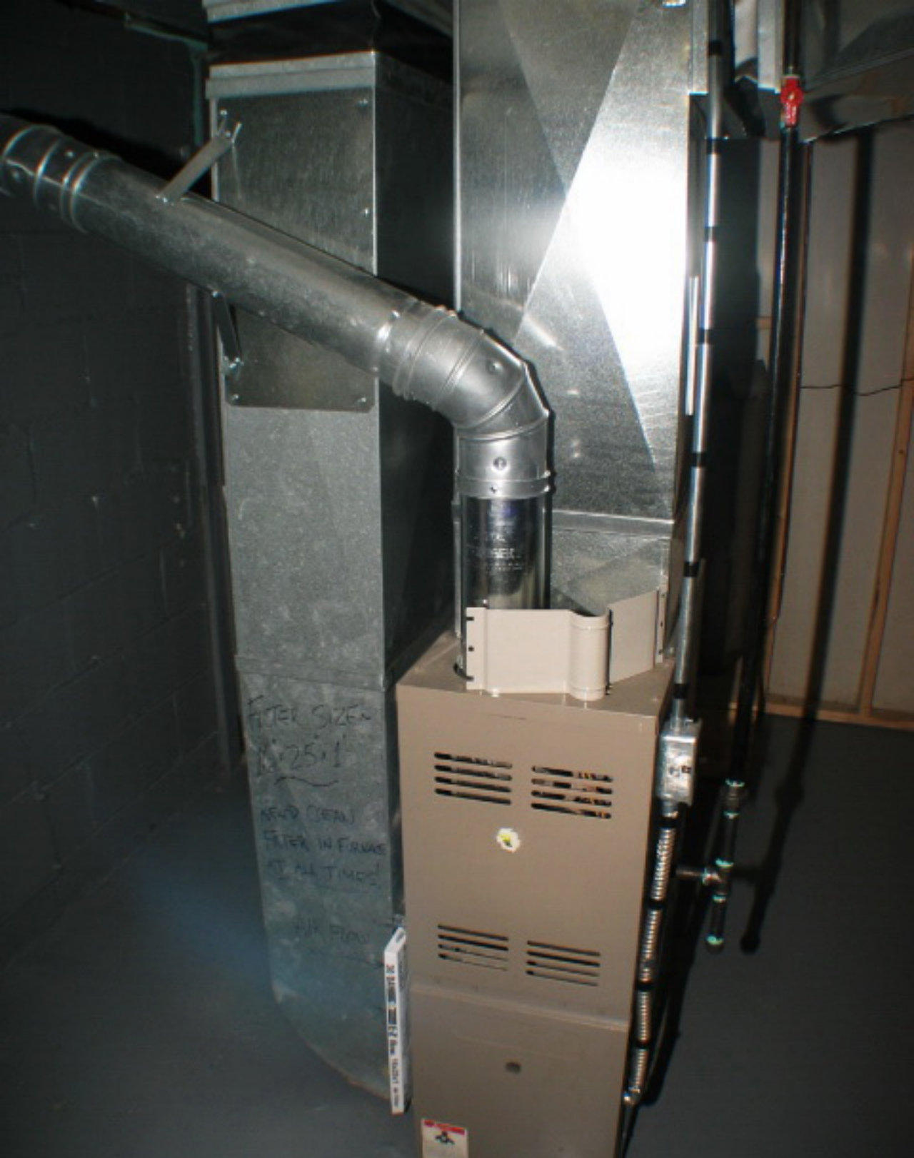
11058 Lakepointe After: Furnace
