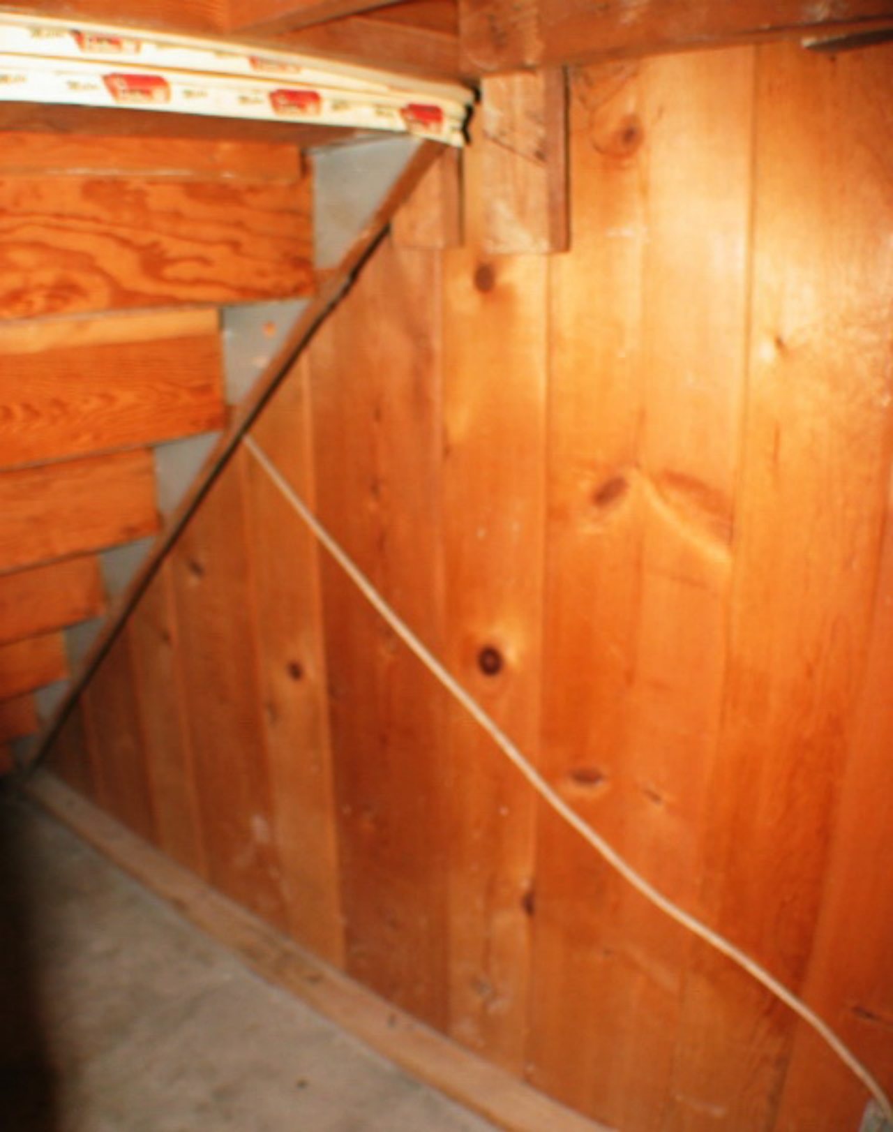
11058 Lakepointe After: Storage1
